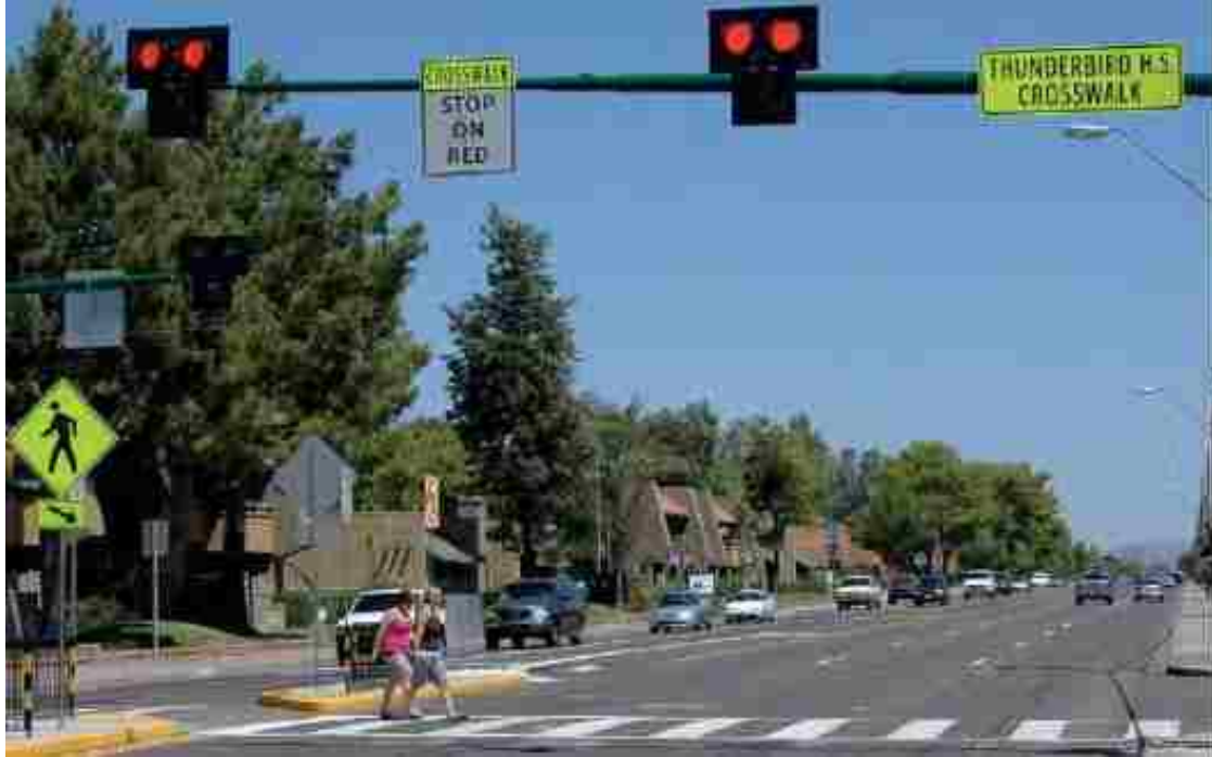
Figure 6-1. A PHB Installed in Phoenix, AZ; note bright yellow signs (FHWA 2014)
